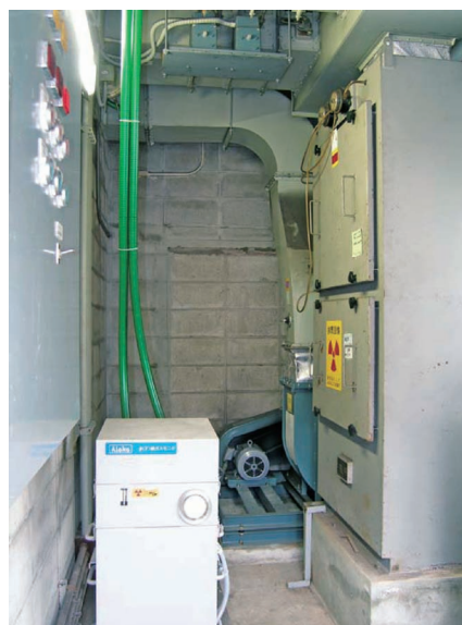
RI exhaust system. All the air released from the RI facilities passes through filters. Air is purified by the filter unit in the right foreground and emitted outside as exhaust by the fan in the background. Radiation level in the exhaust air is constantly measured by the gas monitor located on the left.
